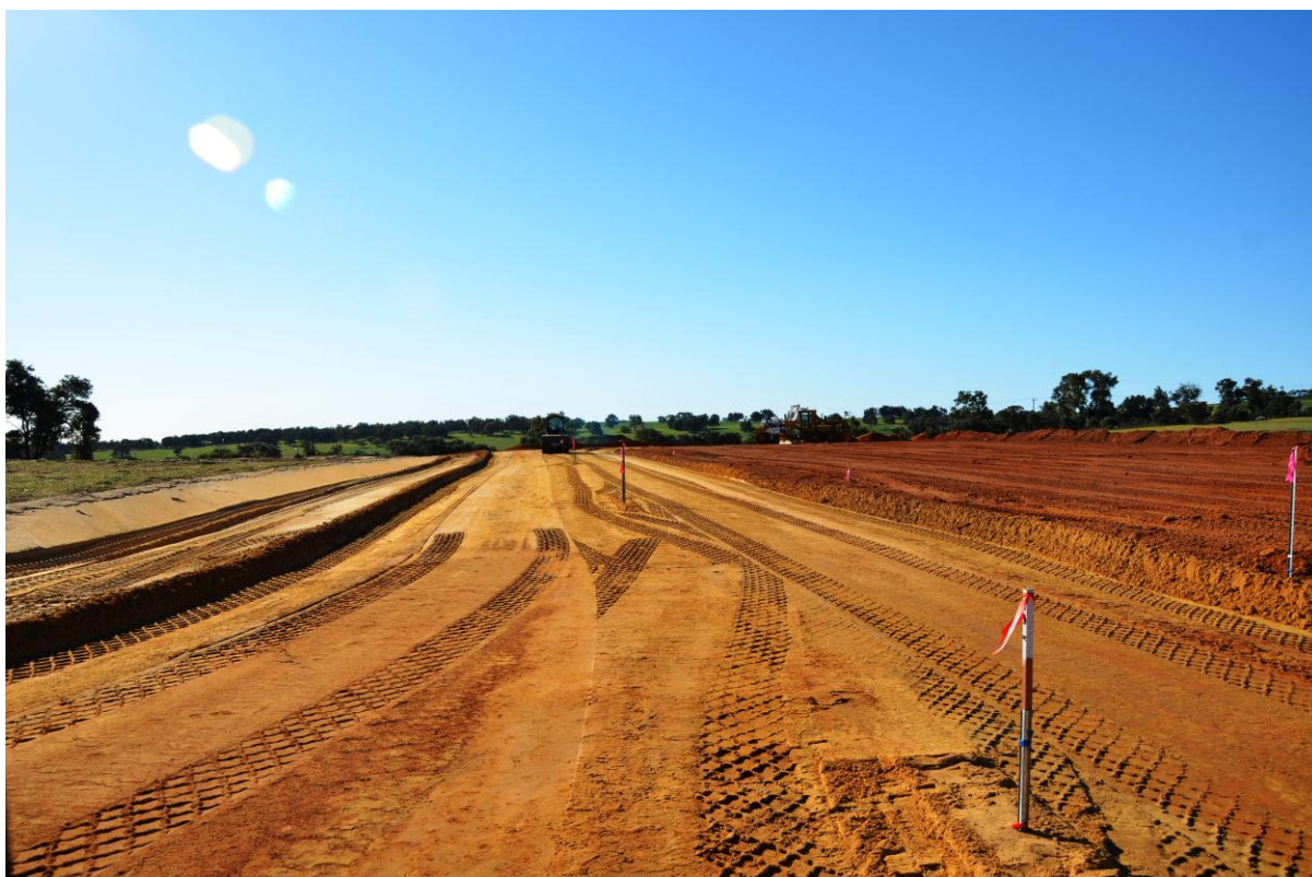
Red Gully Gas and Condensate Processing Facility, 8 September 2012. Centre line (pegged for the ring road) with the Processing Facility hardstand on the right.
