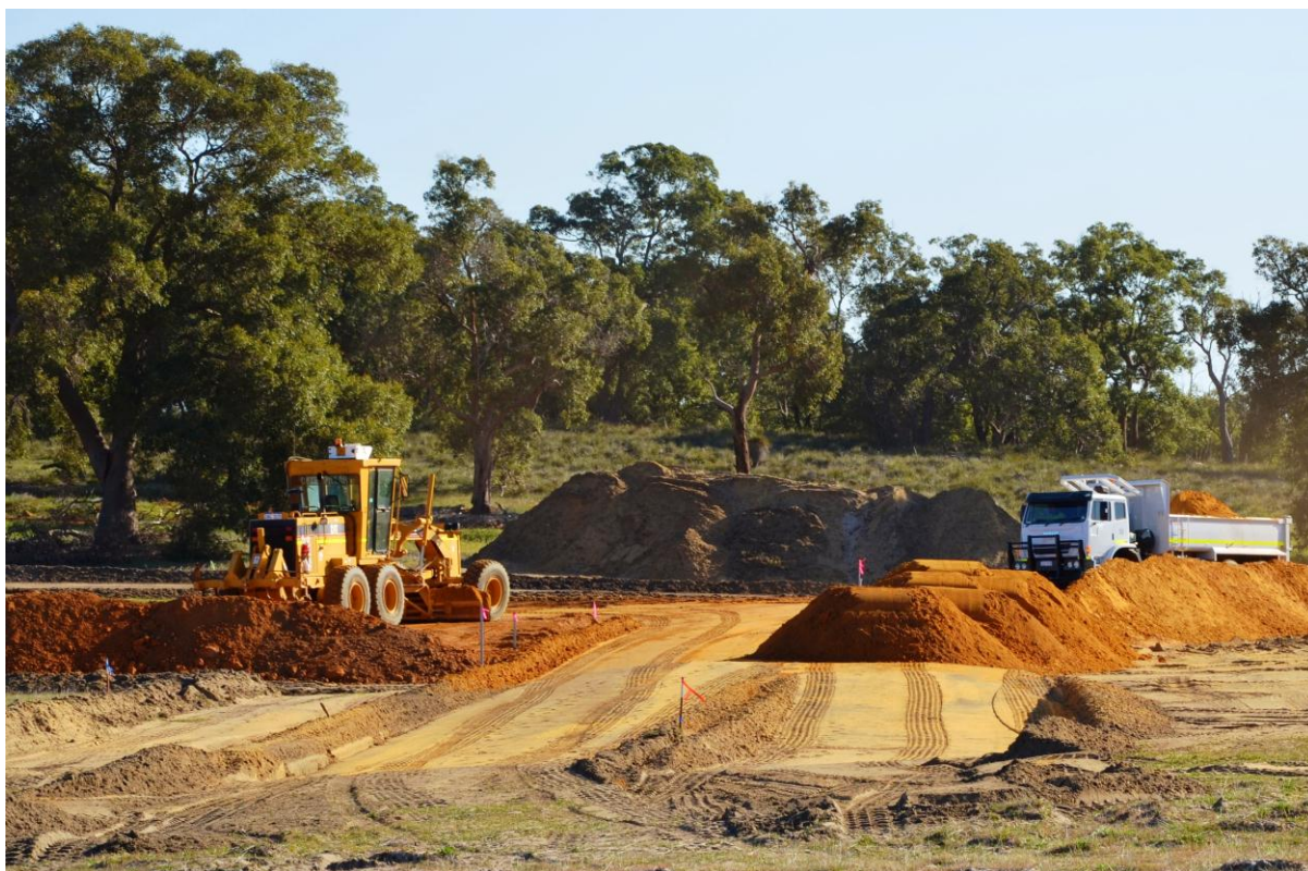
Red Gully Gas and Condensate Processing Facility, 13 September 2012. Commencing gravelling of the site workshop area.
